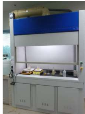
Local Exhaust Ventilation System
