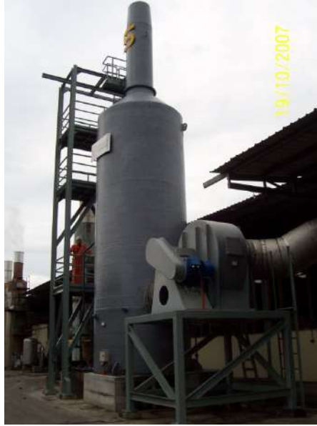
36,000 cfm Odour Scrubber
