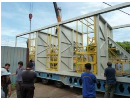
MS Service Tower c/w Staircase
