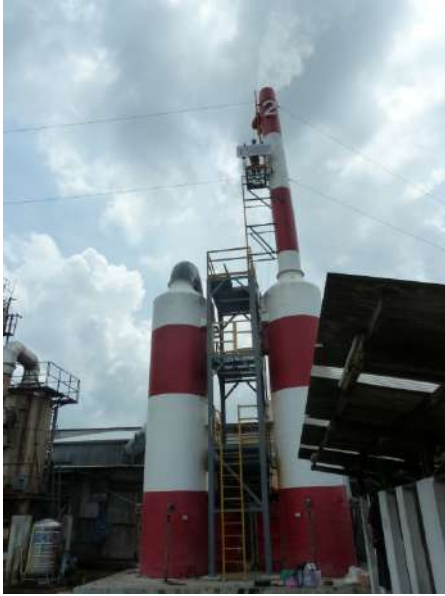
26,000 cfm Compound Scrubber
