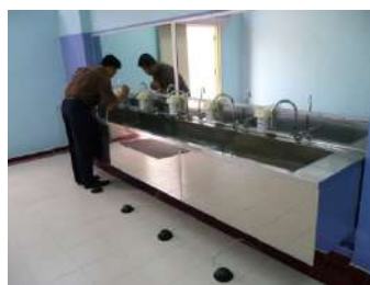
Hospital 6 bay Scrub Sink
