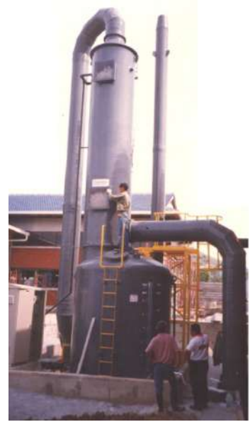
6000 cfm Emergency Scrubber
