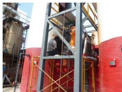
MS/Fiberglass Service Tower
